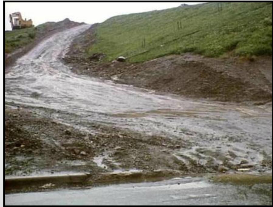
Poorly maintained construction entrance.
