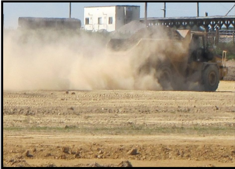
Large area of exposed soils – dust hazard.
