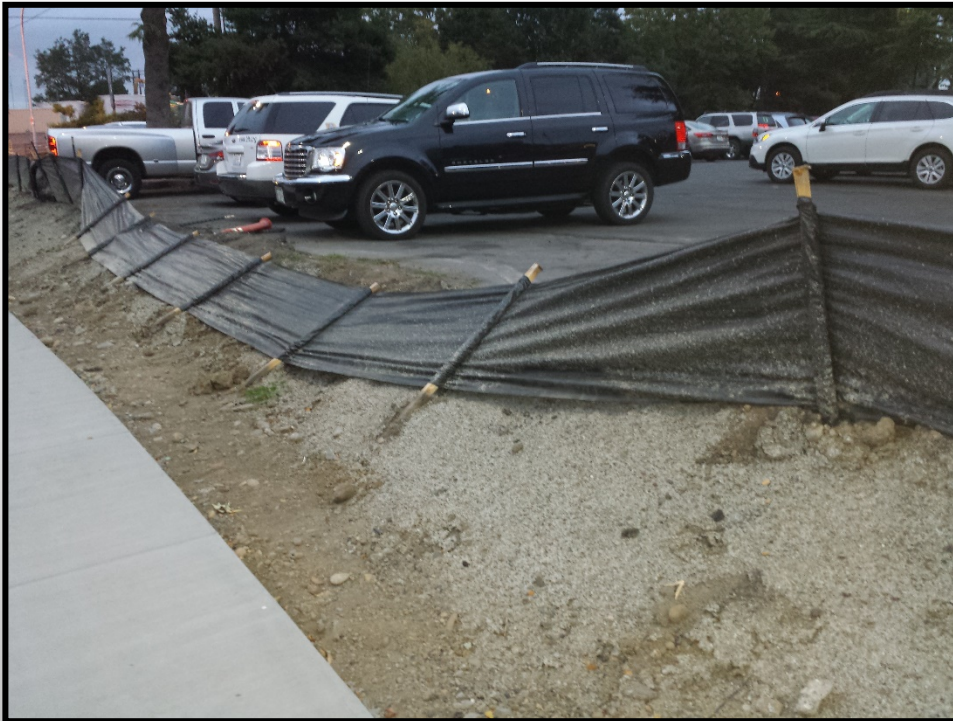
Installing erosion control BMPs incorrectly
