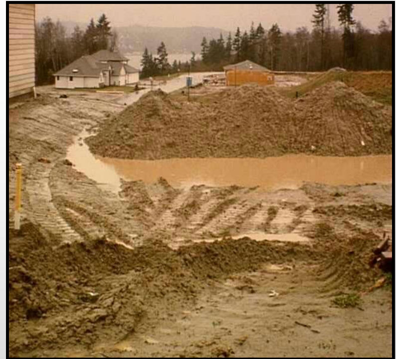
No erosion control efforts
